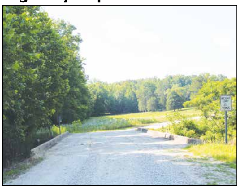
Photo: Work is expected to begin within months to repair the state bridge over Piney Creek on Stack Lane near Silerton. The $300,000 grant received by the Hardeman County Highway Department will foot the bill. Photo by Jerry Rhodes.
